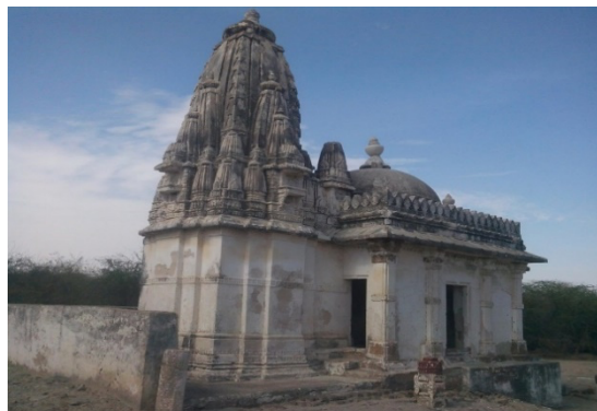
Image 3: (Virawah): Temple's Damaged Boundary Wall
