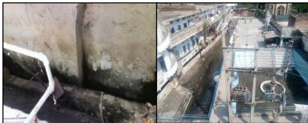
Figure 10: Open Drain and Stream Water Through Gurdwara
